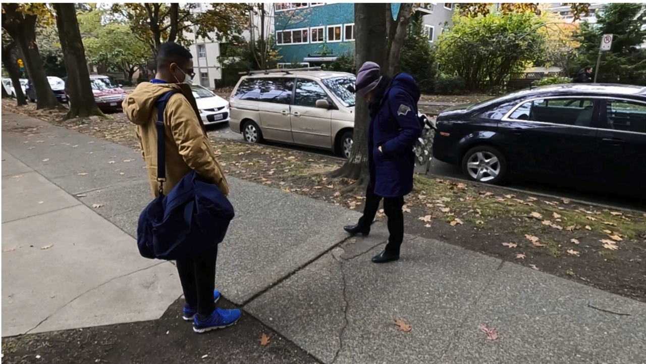
Fig. 4. “I’ve been walking this route for ten years, but still, if [...] I’ve got stuff on my mind, or I’m not thinking, (gestures at joint displacement on sidewalk with her foot) it’s very easy to trip on” (P13).
